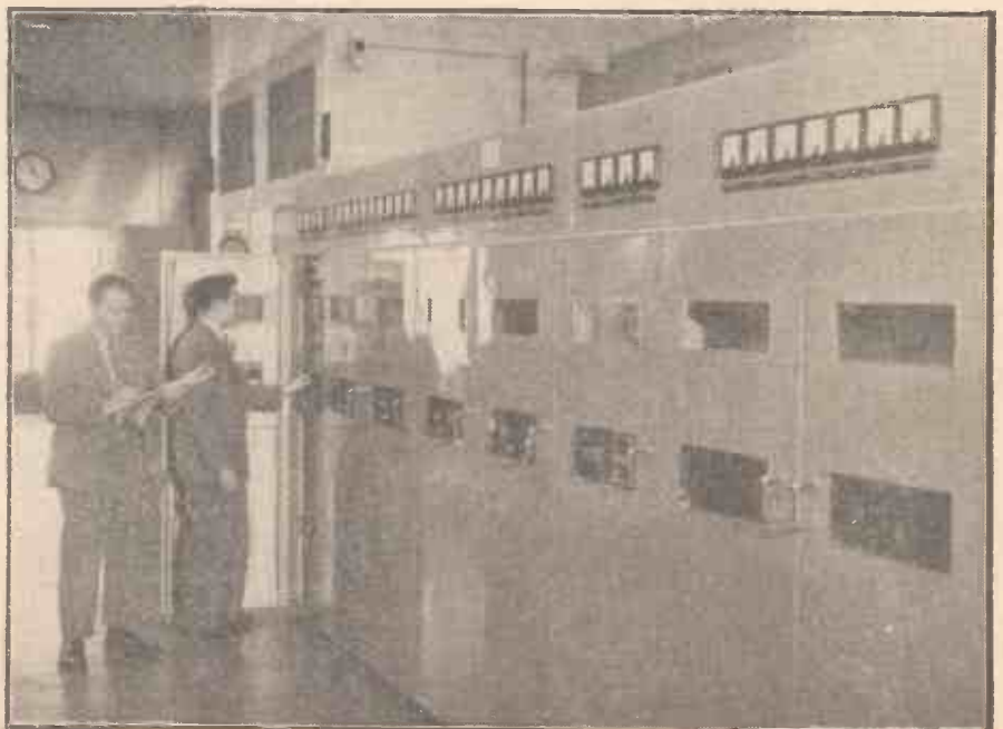
Engineers taking readings at the amplitude modulation (A.M.) transmitter.
