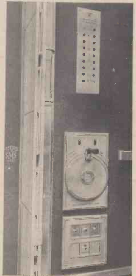
The car control station. In this instance the lift is attendant controlled, a flush-type carswitch being fitted.
