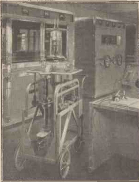
One of the output valves ready for fitting into the transmitter. The valve is carried on a special trolley and is actually wheeled into position.
