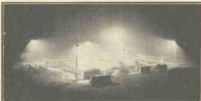
Day-and-night work is being carried out on the extension to the Ekco factory at Southend—an extension that has been rendered necessary by the phenomenal demand for Ekco car-radio installations.
