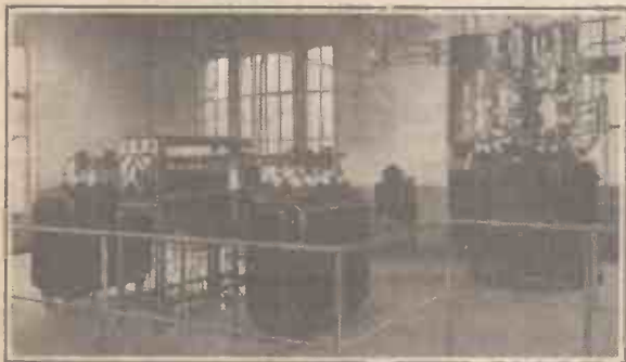
The mercury vapour rectifiers and their controls, and (left) one of the power stages.
