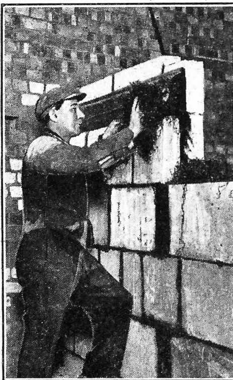
A workman packing the walls of one of the new Portland Place studios with dry seaweed, so as to make them soundproof.
