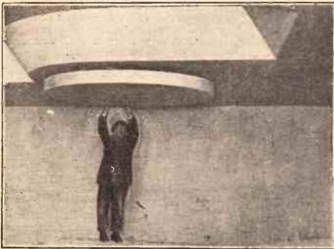
The end of one of the ventilation ducts on the ceiling of a studio at the B.B.C. new Portland Place building. They had a lot of trouble preventing these ducts from carrying sounds from studio to studio.
