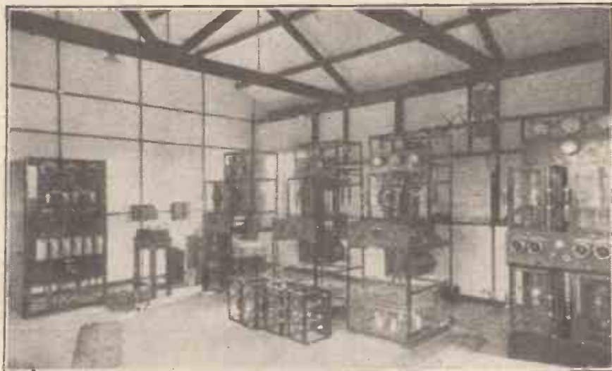
The valve panels in the transmitting room at the Durban station.
