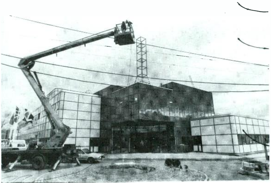
Newcastle's £10 million regional broadcasting centre was topped out during the year. The centre will provide a home for Radio Newcastle as well as regional television in 1986.
