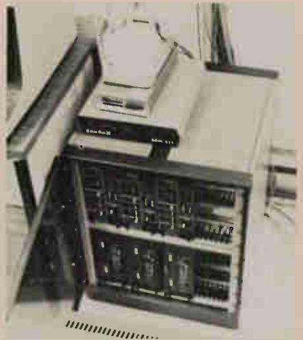
Three 24-channel multiplexers and three SM 9600 superModems are part of data-com equipment. LDM 414 unit on top of cabinet supports communications between Victoria headquarters processors with CRTs at Swartz Bay, 17 miles distant.
