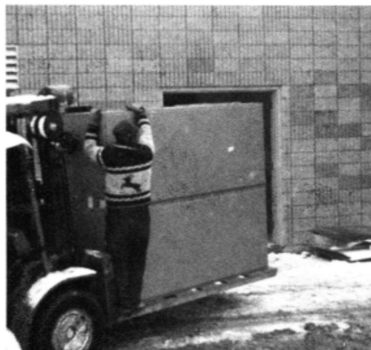
The visual cubicle of the transmitter aided by Joe Leclerc of Townsend Associates being rolled into the building. Note the "muck" stirred up by all the activity.
