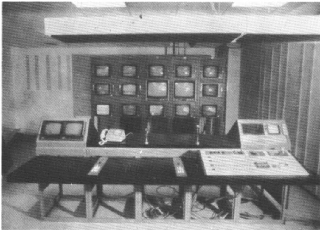
Studio control room
