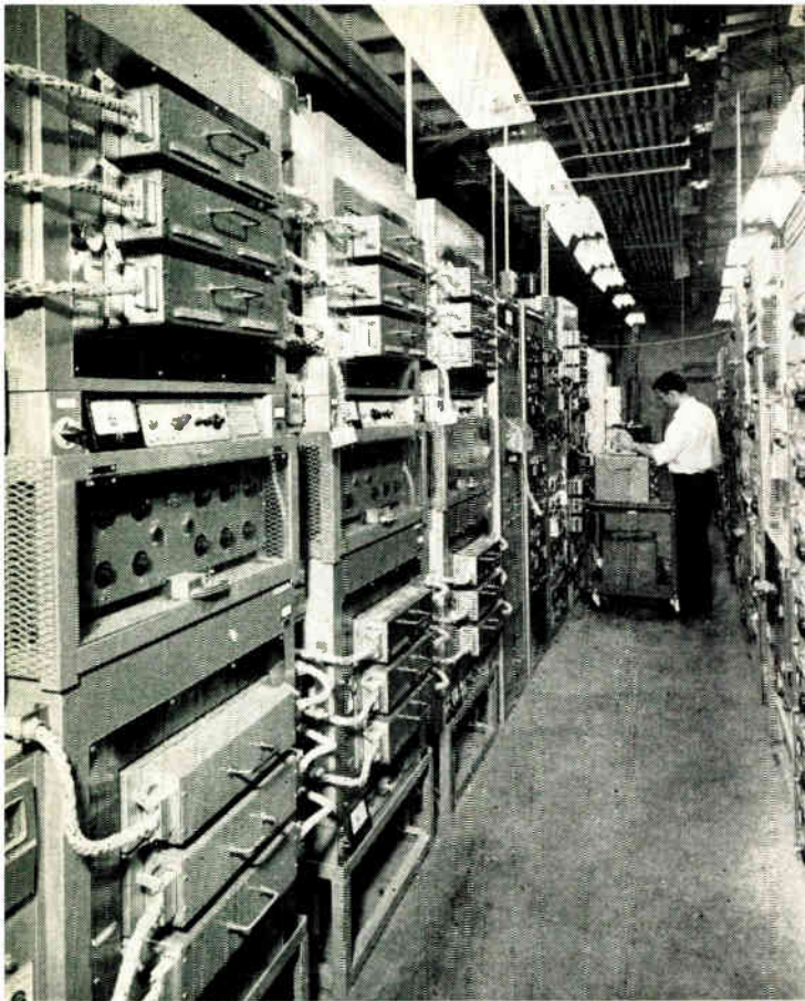
View of the test installation shows the capacitor test ovens on the left and a bank of variable resistor test chambers on the right.
