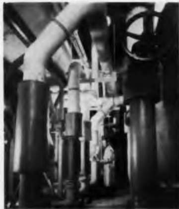
This 6,400 square foot service area at Raytheon's new Lewiston, Me. plant supplies all the utilities required for modern semiconductor production.
