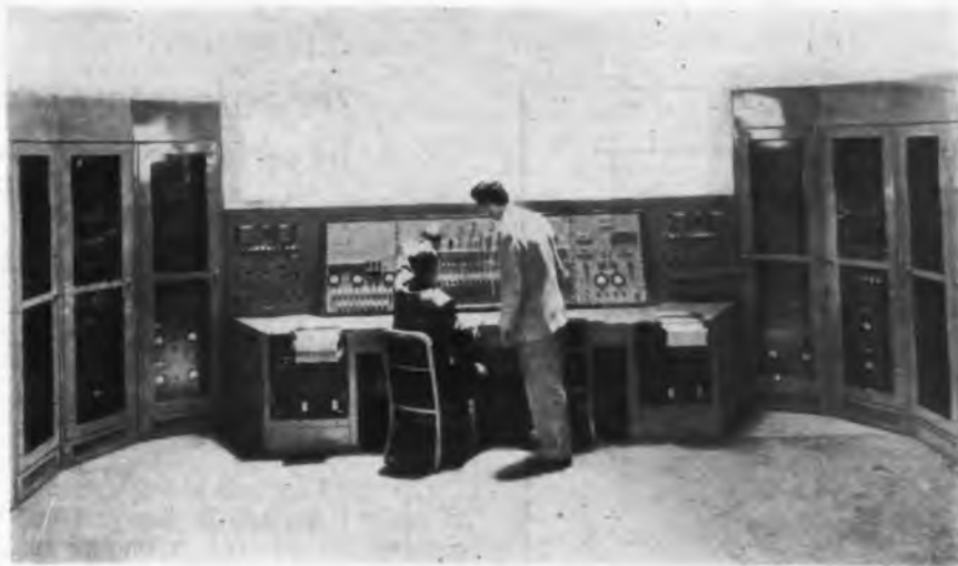
Fig. 1: Dual Timing Signal System installation at A.F. Guided Missile Center, Cape Canaveral, Fla.
