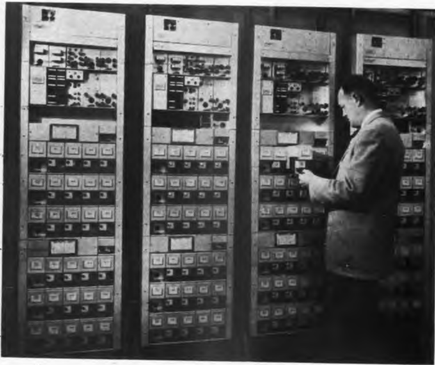
Fig. 1: Two complete 48-channel terminals for Type 45BX system for multiplexing wide band radio
