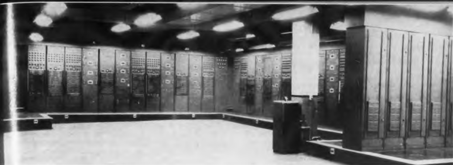
Fig. 1: Computing equipment in Project Cyclone Simulation Lab. Power supplies and voltage regulators are located in room behind laboratory
