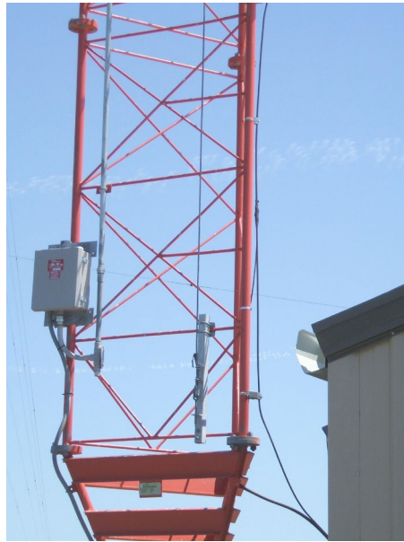
One of the WOR-710 towers, showing the wiring necessary for the aircraft warning lights. (Doug Smith)
