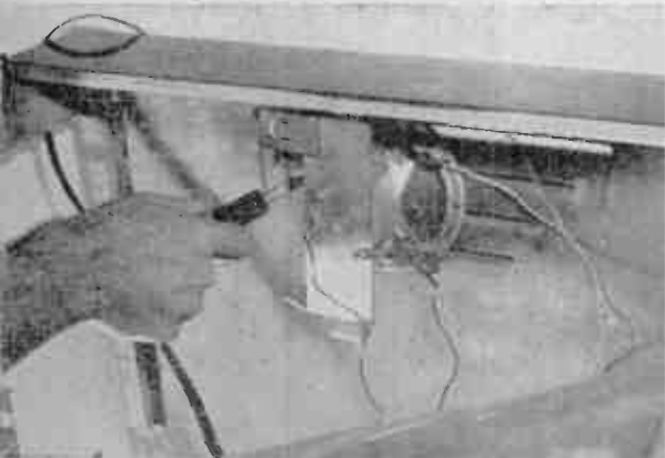
18 After set was pushed into cabinet I re-mounted the speaker in its new location, frame and all. Leads have to be extended, and it's essential to ground speaker frame to chassis.
