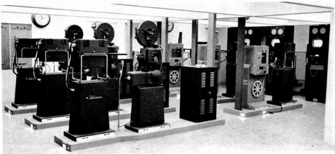
Fig. 11 The telecine room employs a separate film camera with each projector. A standardized rack of equipment associated with each projector-camera grouping contains all audio and communication facilities, as well as picture monitoring facilities.
