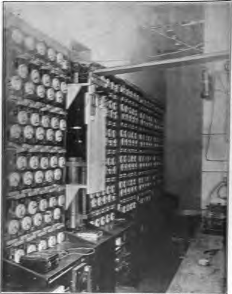
FIGURE 8—Power Tube Racks, First Group
