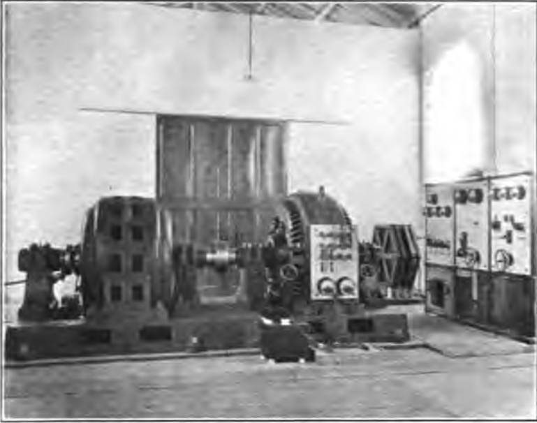
FIGURE 5—Motor Generator and Control Panels, Rome Radio Station
