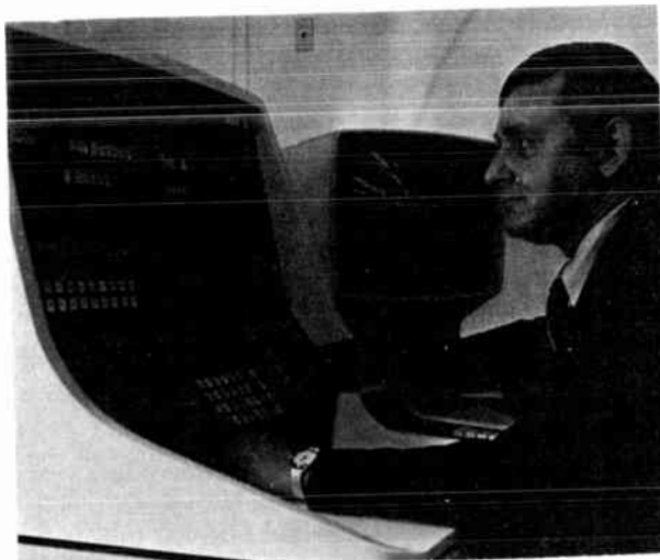
[2] Toll test desk for the North Electric Co.'s ETS-4 large-capacity telephone switching system in full operation.
