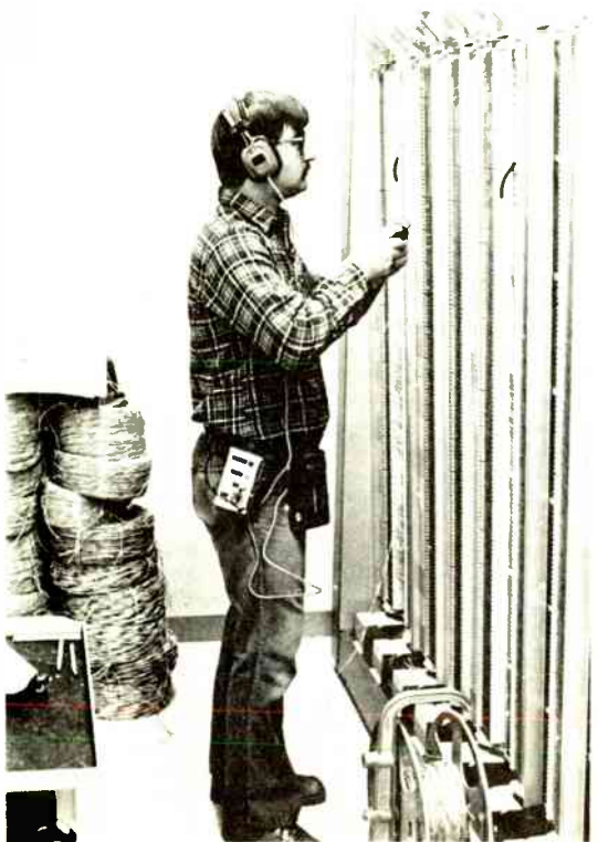
[B] Headphone instructions are received by this telephone installer from a belt-secured cassette player.
