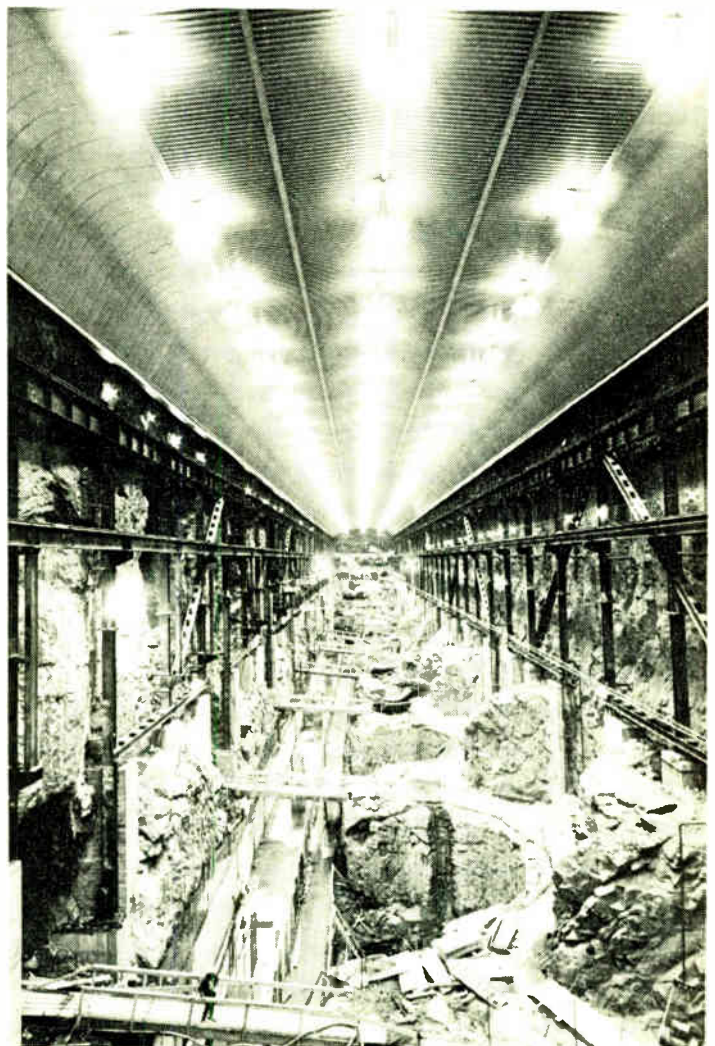
FIGURE 14. View of the powerhouse after the completion of excavation. This underground chamber, which will be the world's largest generating facility, is situated about 300 meters below grade.
