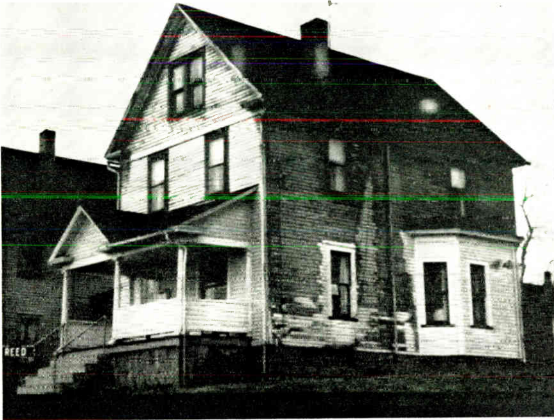
Fig. 8. Paint damage caused by air pollution. In this case, the pollutant was hydrogen sulfide.
