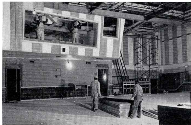
FIG. 10. WCAU STUDIO IN THE CONSTRUCTION STAGE, SHOWING NOVEL USE OF ACOUSTIC BLANKET
