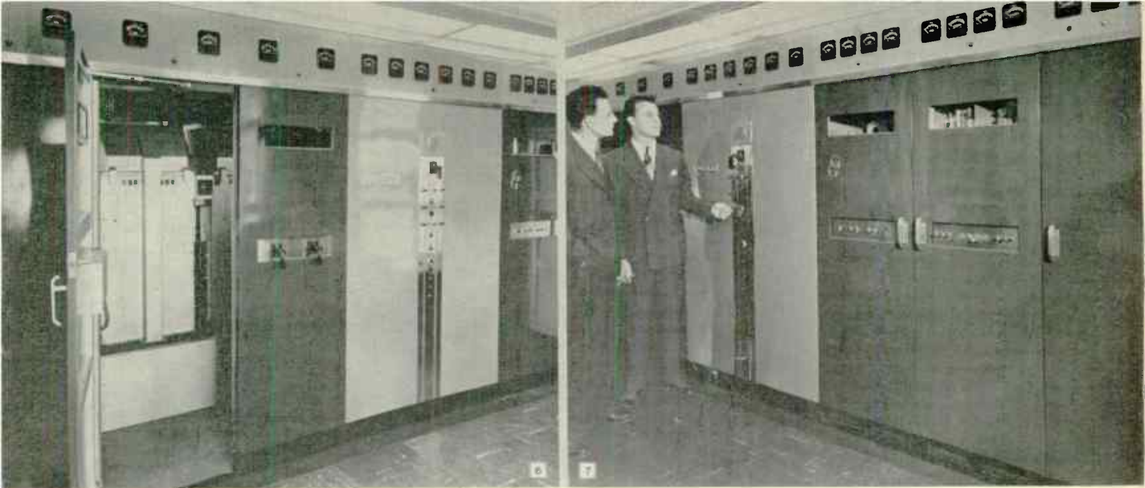
Fig. 6 Output end of the transmitter panel. Fig. 7. Modulator and driver section. Fig. 8. Close-up of the 50-kw. output amplifier.
