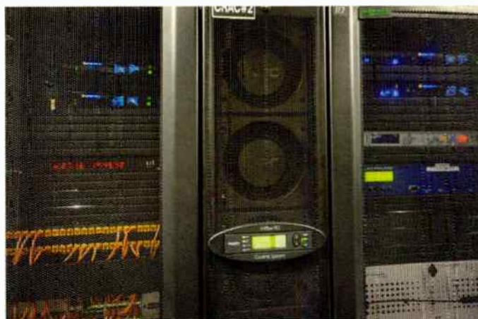
Rackroom gear is cooled directly at the source.
