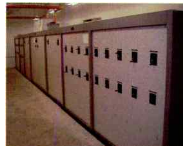
CUSTOM PHASOR INSTALLATION
