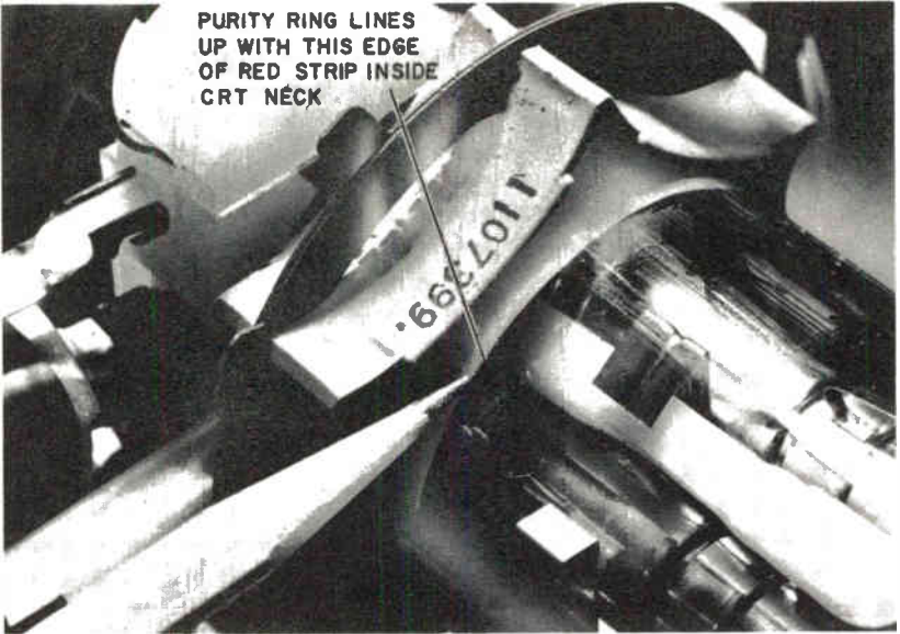
Fig. 407. Center purity ring is lined up with the red stripe on the neck of the CRT.
