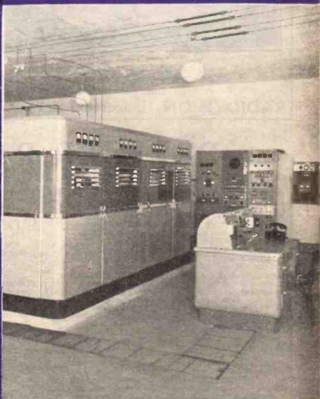
The transmitter room at "Busto Arsizio", Milan.
