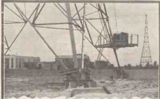
The foot of one of the masts of the new transmitter
