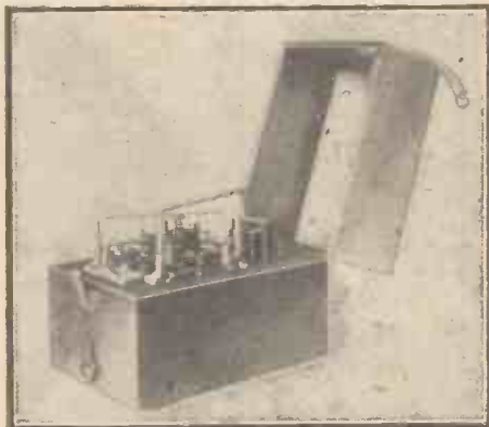
Fig. 3.—An Unusual Method of Wiring carried out by Mr. J. E. Bates, of Coventry.
