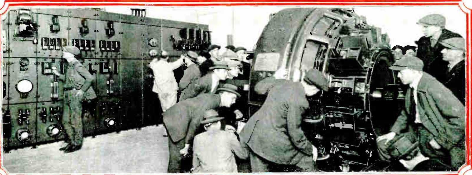
This is an automatic substation of the street railway systems, and the students are shown examining the 2000 K. W. converter, and switchboard. Trips to such plants as these are intensely interesting.
