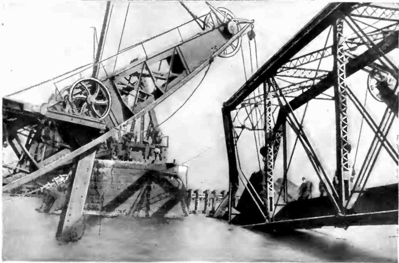
Two Views of a Remarkable Piece of Repairing by Railroad Engineers. The Span of the Bridge, Which Was Pushed Off Its Masonry Foundations, Was Put Back Into Place by Means of Two Steam Dredges and Two Old Scows.
