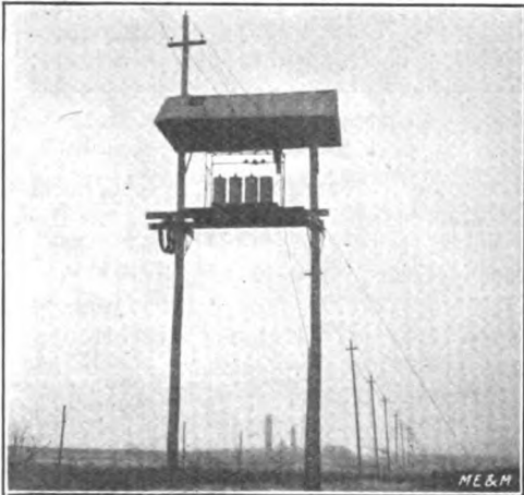
THE LAND END OF THE TRANSMISSION LINE, SHOWING THE TRANSFORMERS
