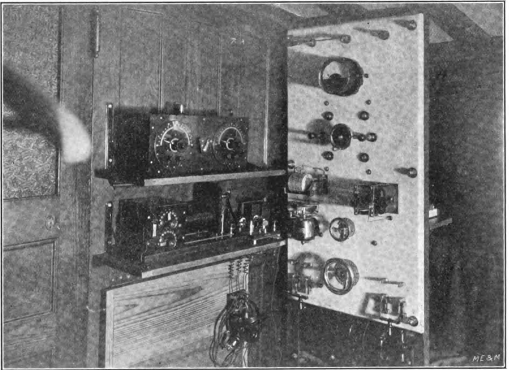
THE WIRELESS EQUIPMENT OF THE "TARRAGON," SHOWING THE RECEIVING APPARATUS AND CONTROLLING SWITCHBOARD.
