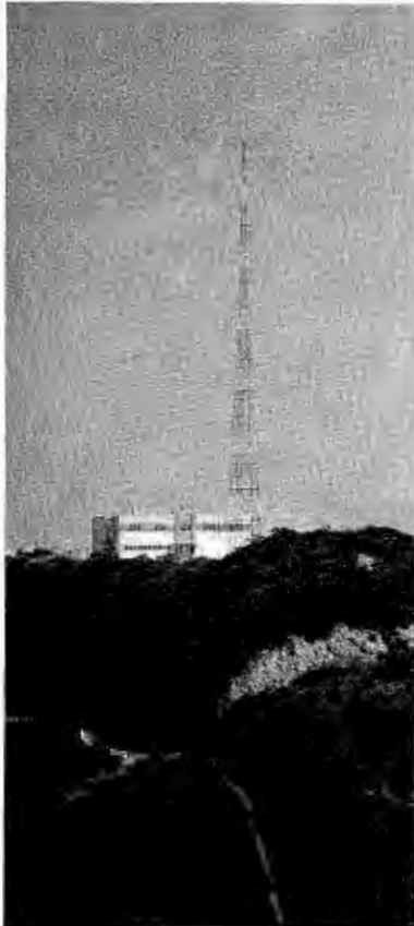
The Mt. Lee television installation. This is the receiving location for all portable pickups.
