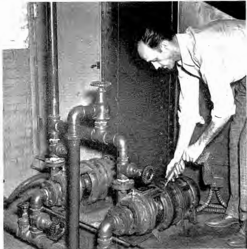
Figure 2 Greasing a pump motor with a hand-operated grease gun.
