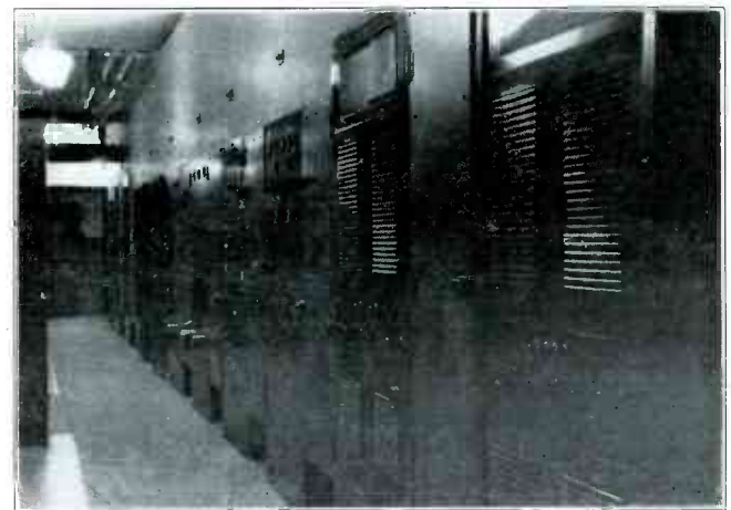
View of W2XBS Transmitters. Portion of side Band Filter can be seen near ceiling.
