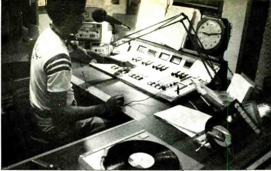
FM studio has turntables to right of operator for origination of all programming from discs; DJ Clifford Brown Jr. is on air. Remote control and status units are in racks behind him
