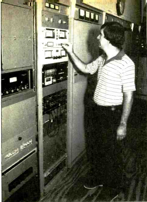
In transmitter room, chief engineer John Francioni adjusts the receiver for the UHF repeater signal, coming from mobile units. Transmitter is to his right
