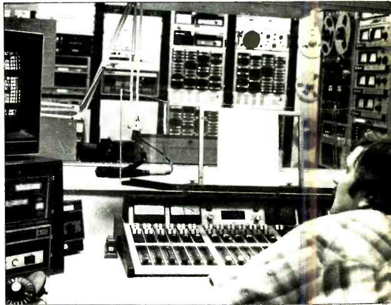
Lamb is at console in studio A, with automation systems in front of him and to his right in main control room beyond window
