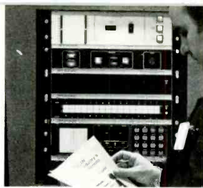
TFT's microprocessor remote control system continues to expand its capacity
