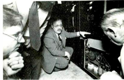
Harris TV transmitter gets close inspection by broadcasters.
