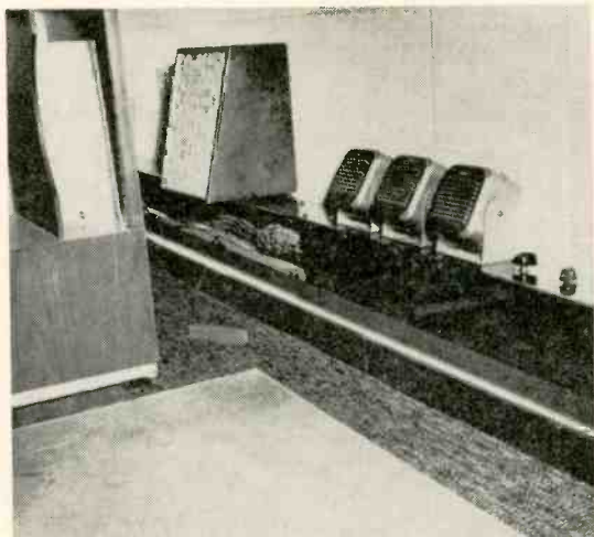
View of wiring duct near master control console desk. Utility speakers are for mobile, EBS, and talkback; 8" baffle mounted speaker is house monitor (console monitor is theatre-type speaker).
