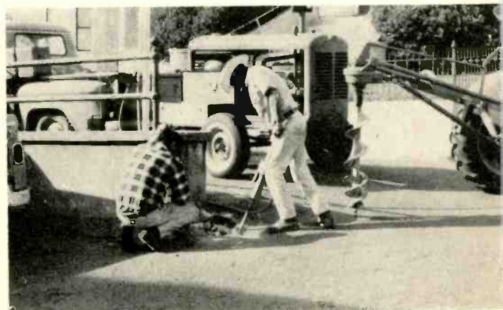
Earth-boring equipment and air hammer, powered by mobile generator, are often required when setting your own poles.
