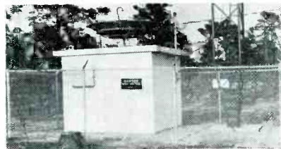
CATV head-end equipment housing at base of tower. (Note microwave dish on top of building.)
