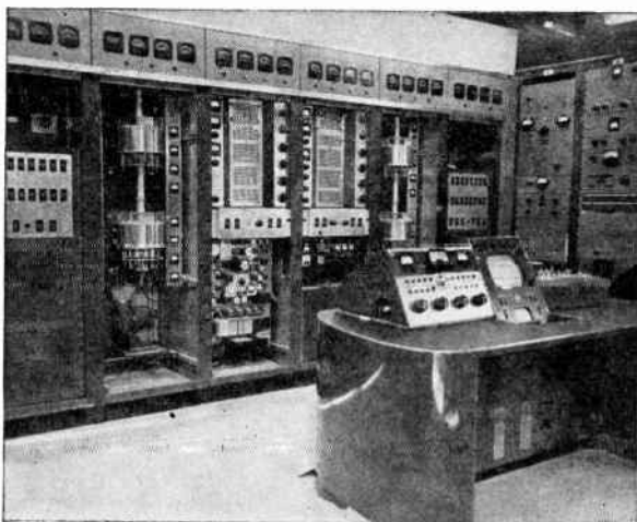
Fig. 8—The RCA TTU-1A transmitter, input and monitoring racks and control console.
