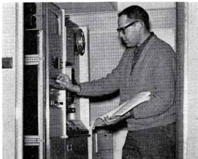
Leonard Gostin, station engineer, checks TR-4.
