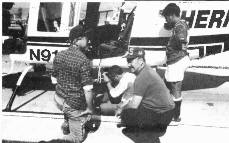
Ron WB6FXW, Bob W6LUY and Hector (the mechanic) install the ATV antenna on the helicopter. Rick N6ZT shooting video of the activities.
