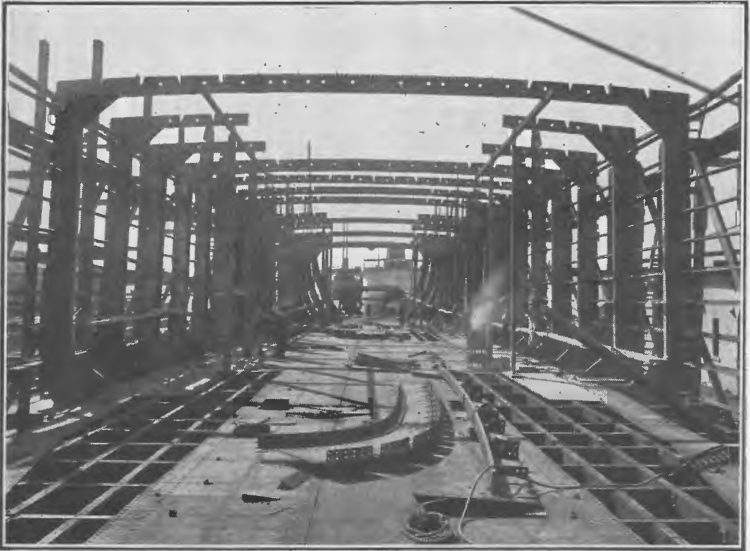
"Commonwealth Ship No. 1" at the End of August, 1918, Showing Longitudinal and Transverse Framing in Position.
