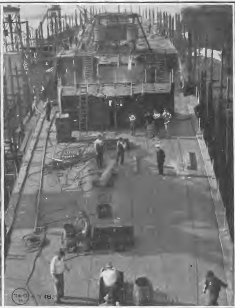
July 4, 1918.—General Deck View Showing Searchlight Platform (228th Day). Note Lines of Compressed-Air Riveting Machines.
