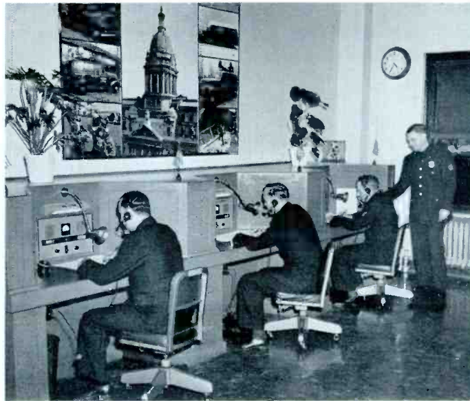
Two-way radio communications system installed for the Brooklyn, N. Y., police department uses RCA equipment.
