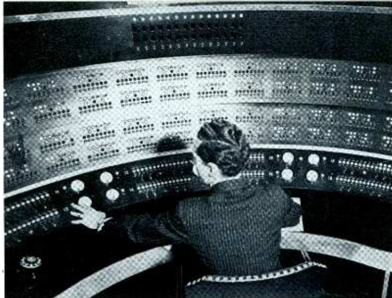
The master control board in Radio City with its myriad switches and flashing lights is the nerve center of the NBC network.
